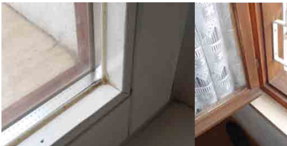
Figure 5: Existing double glazed (left) and single glazed (right) windows [ZEPHIR 2013].
