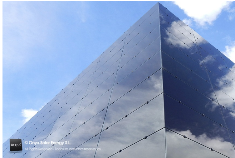
Figure A2: Photovoltaic ventilated façade (a-Si technology). The Black Box, Ávila (Spain). Source ONYX
