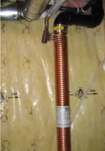
Figure 30: Installed drain water heat recovery pipe © Wagner Solar
